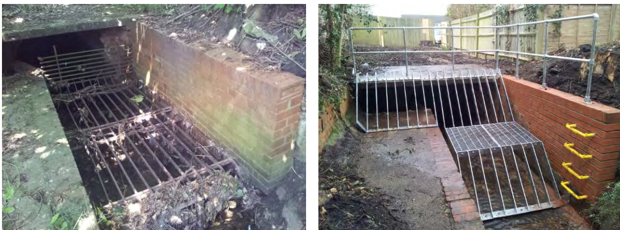
Figure 2-3 Orion Car Park trash screen in June 2015 (before – left) and April 2016 (after works completed – right)
